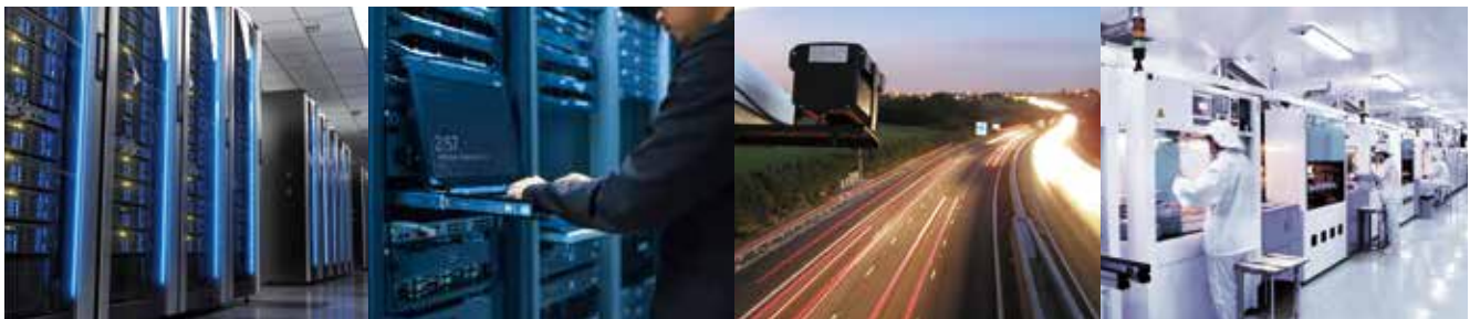
Enterprise Data Center
